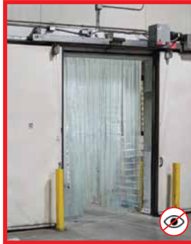
BLOCKED LINE OF SIGHT WITH PLASTIC CURTAINS
