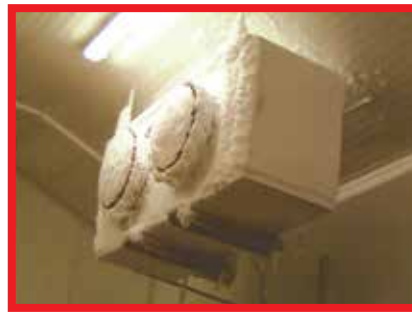
FROST BUILD-UP BEFORE AIR BARRIER INSTALLATION
